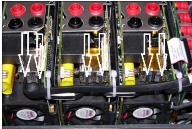
Figure 120 Communication Cable Connections
