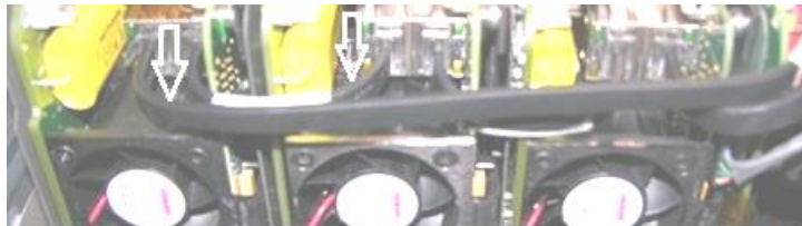
Figure 156 Communication Cable Connections 3 Channel Unit
